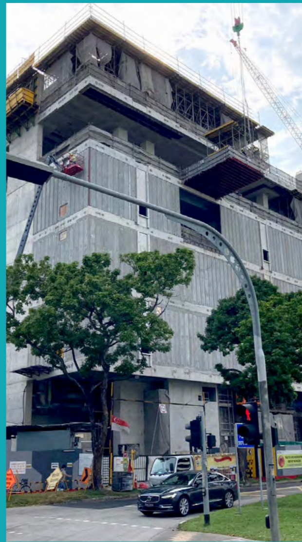
STTelemedia Global Data Centres at 51 Defu Lane 10
