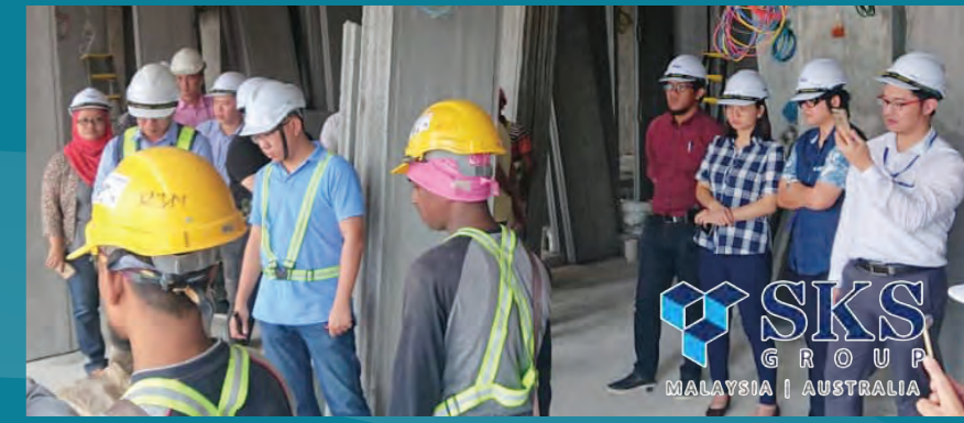
SKS Group and Atria Architects visit JOE Green's project site Holiday Inn JBCC
