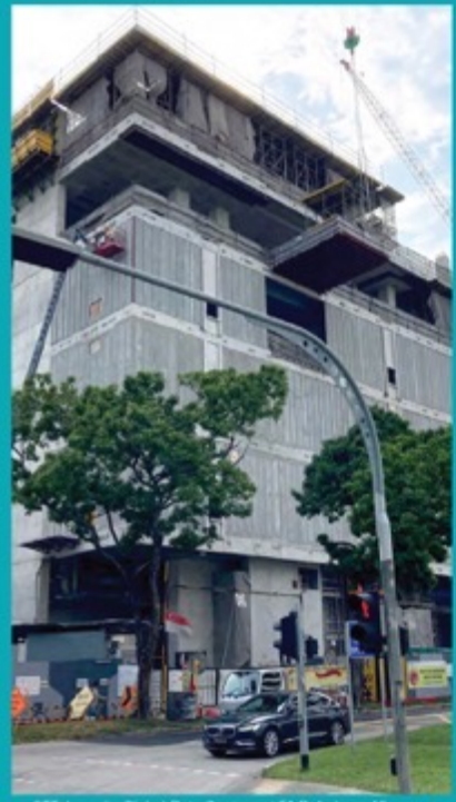
STTelemedia Global Data Centres at 51 DeFu Lane 10
