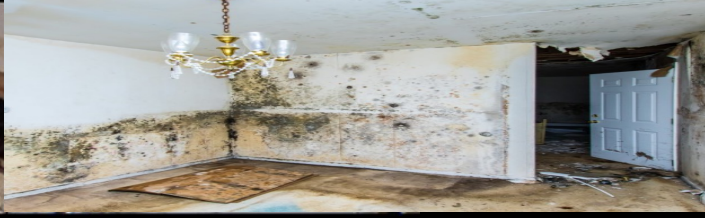
Mold and Fungus
