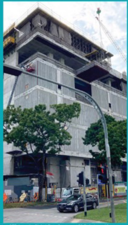
STTelemedia Global Data Centres at 51 DeFu Lane 10
