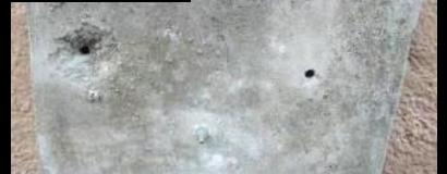
Susceptible to Cracking (Vibration)
