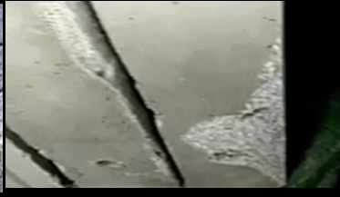
Joint Crack and Peel Off
